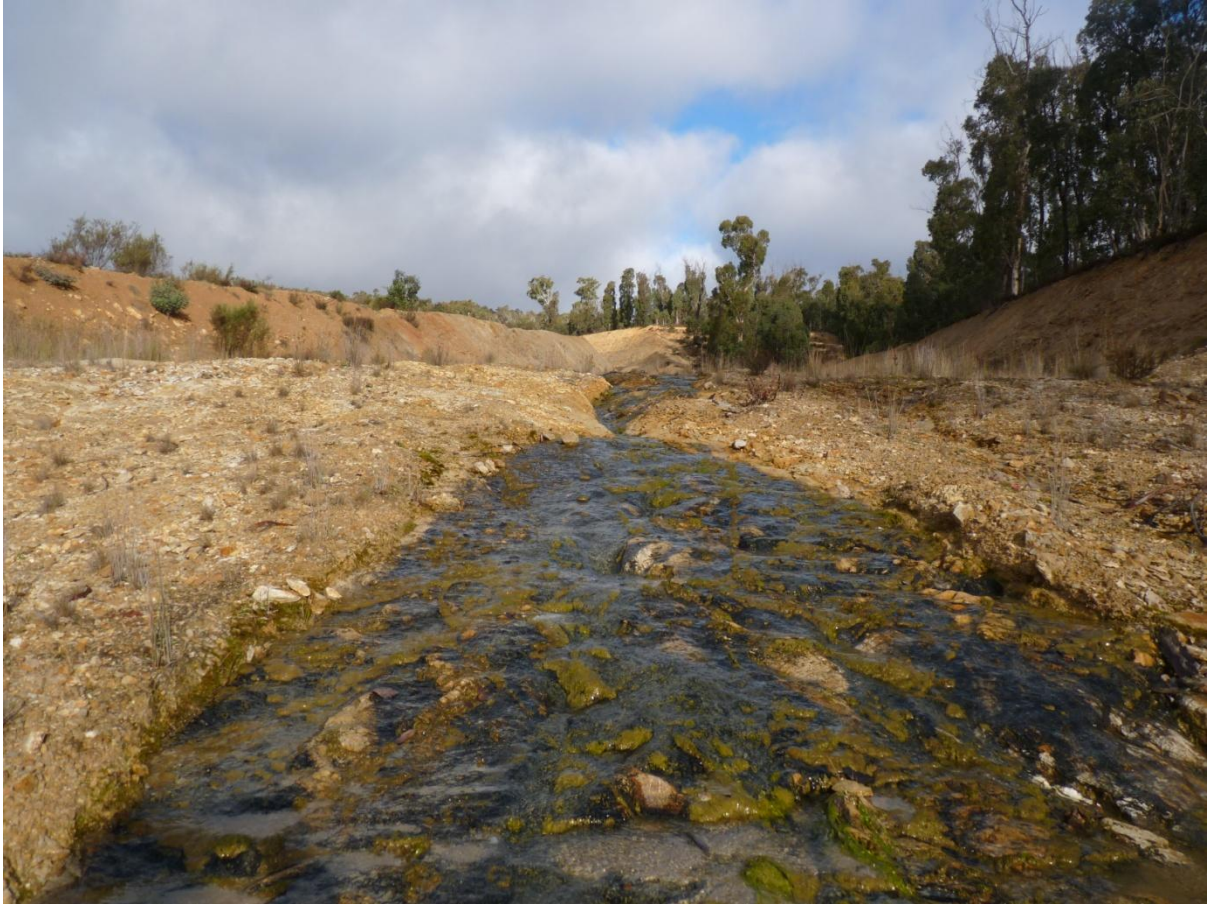
Tailings dam spillway seepage #1
