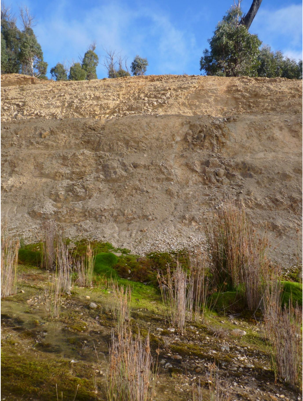
Tailings dam spillway seepage #2
