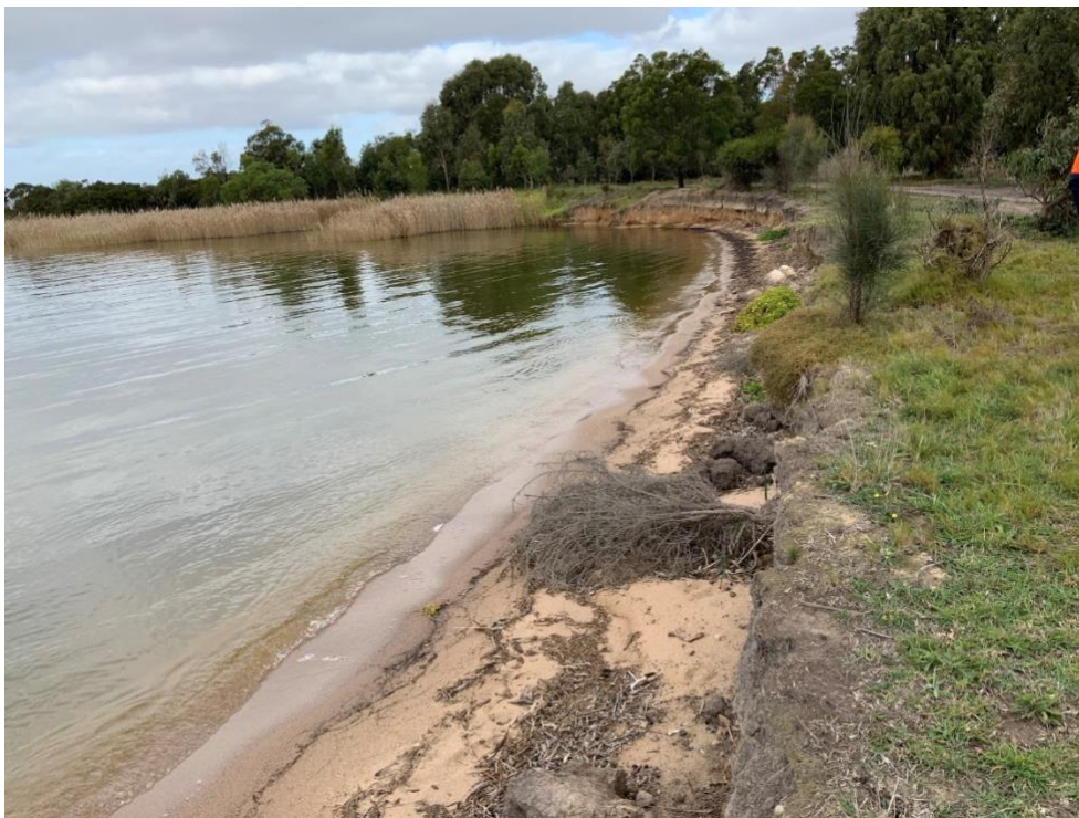
Salt laden water high above the usual water line is very damaging to vegetation. At Marlay point waves went over the concrete wall and eroded the infrastructure.
